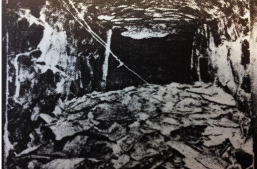
Figure 78. Thermal spalling in an exhaust gas drift at North Bay, Ontario (Lee et al., 1982, p. 964).
